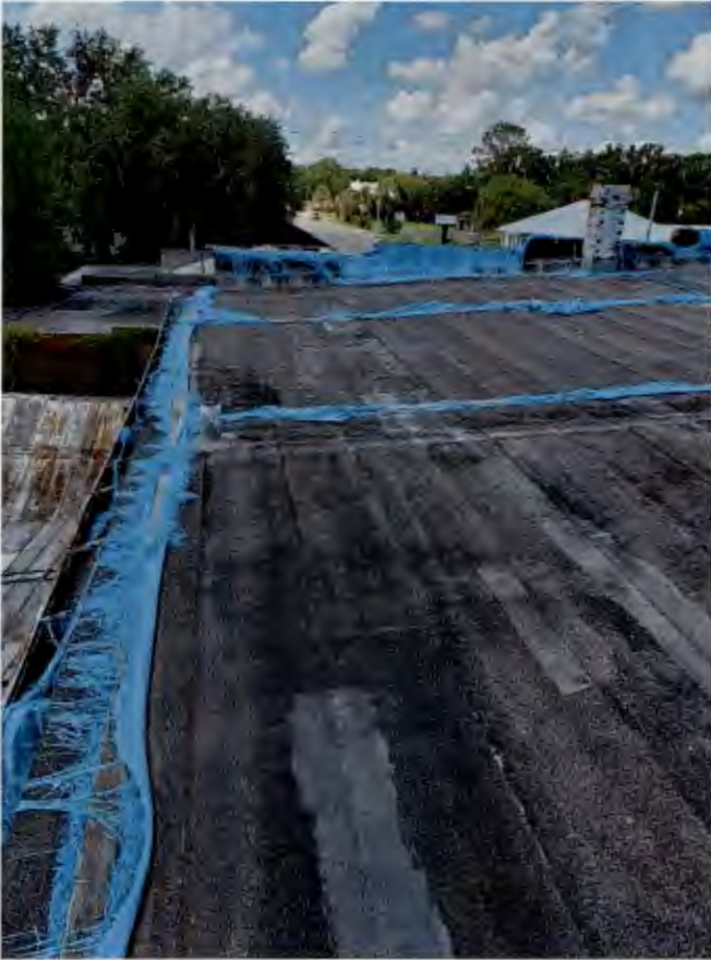
Photos 4-6: Roof Deterioration, Garage Main Building and Gabled Wing (East)
