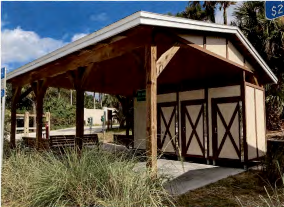
Pedestrian Changing Building- Constructed in 2016. No visible damage. No paint chips. Roof and eaves are in great condition.
