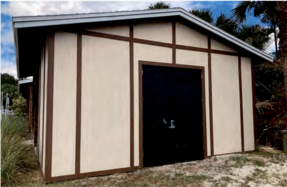
Storage and Pavilion Area- Constructed in 2016. No visible damage. No paint chips. Roof and eave are in great condition.
