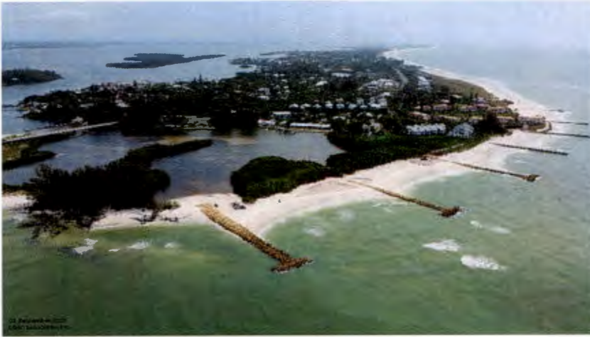
Figure 3 An example of structural stabilization along an inlet shoreline. The image depicts the construction of low-profile rock groins, prior to filling of the structural groins at Longboat Key with beach-compatible sand.
