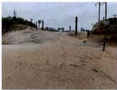
Pre-Construction Eroded Conditions
