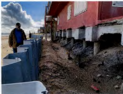
Eroded Pre-Construction Conditions (2018)
