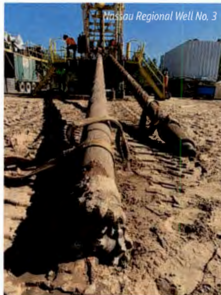
Our proven, streamlined approach to wellfield DB delivery can reduce the time of completion from NTP by 50%.
