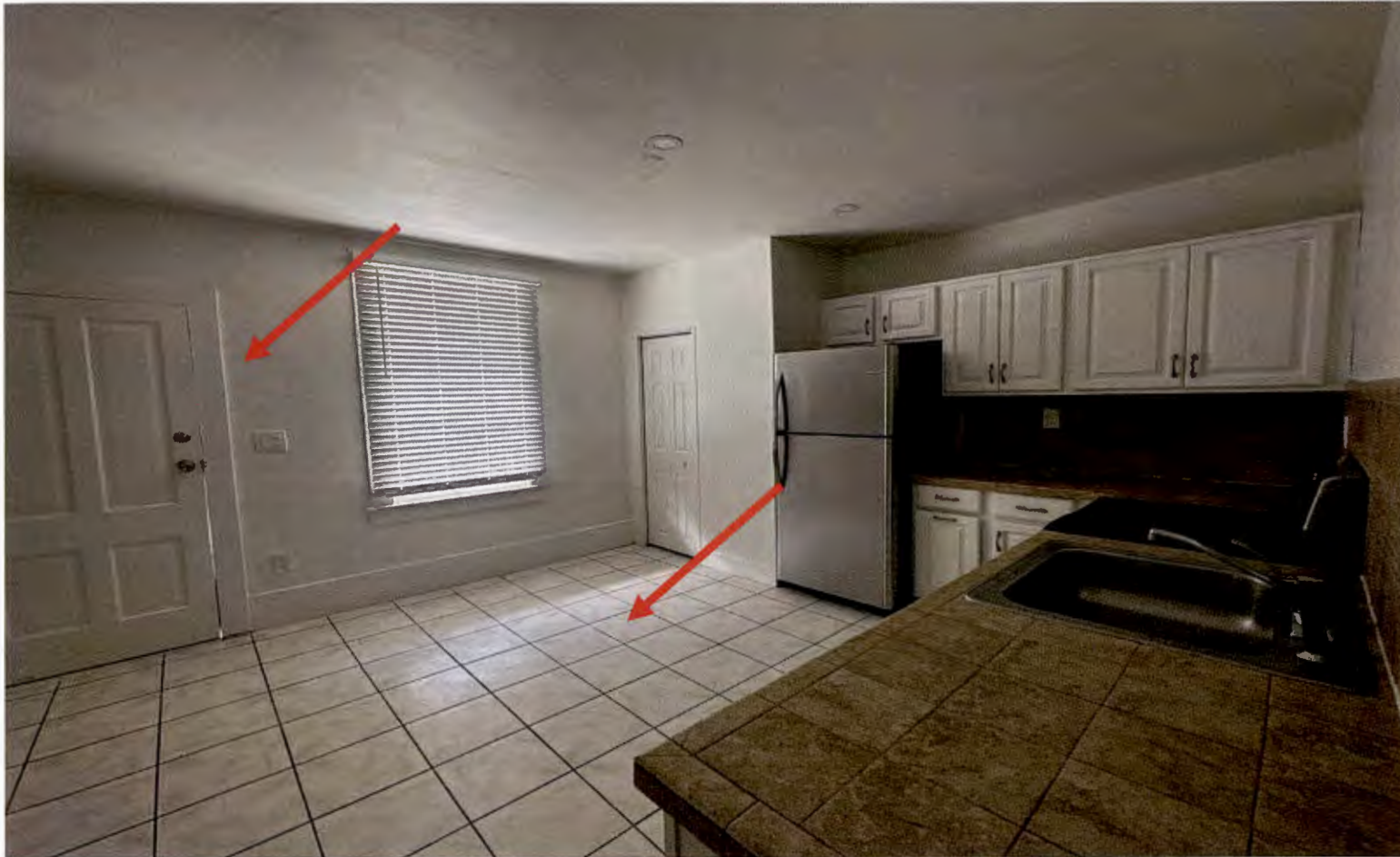
PHOTO 7-6: APARTMENT 1-KITCHEN, PRESERVED FEATURES: FACING WEST Updated version Received December 13, 2023 Planning & Building Department
