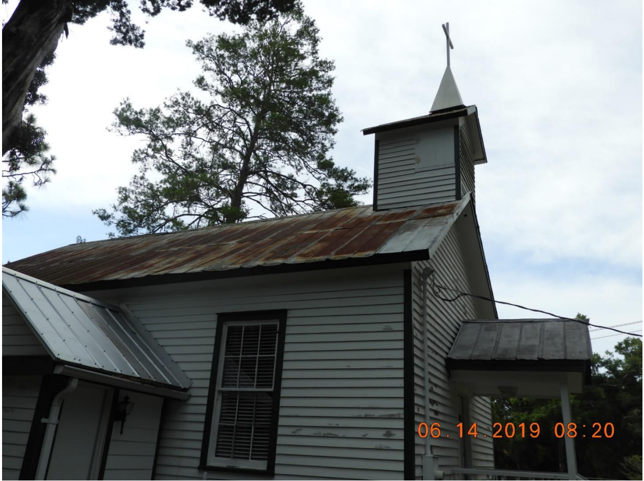
Figure 7 Roof on addition has been replaced, roof on front entry has been painted, but the main roof has not been replaced since 1941.
