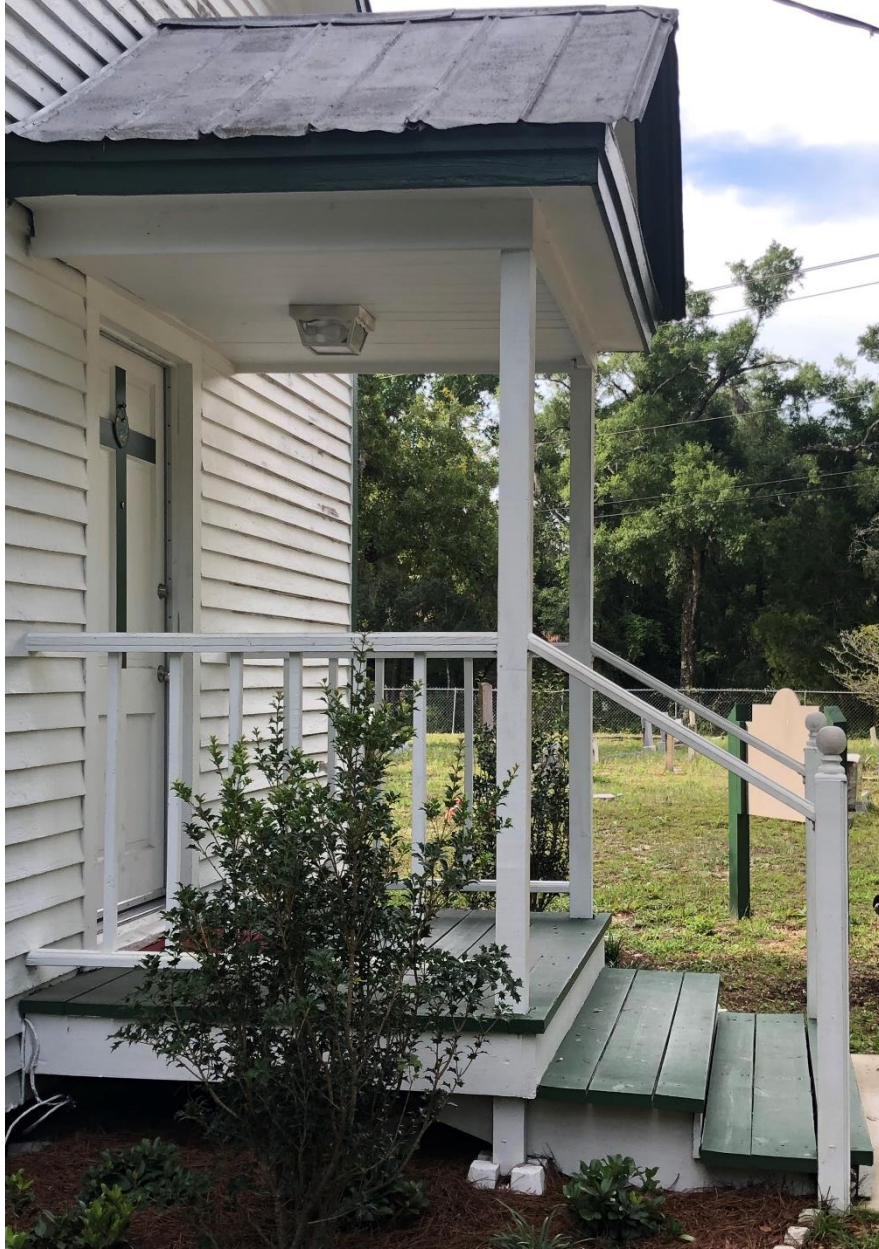
Figure 8 During the June 17, 2019 site visit, Nick Jonhakis noted that the front entry porch may have been an addition to the original building. According to images in newspaper articles, the addition has been in place since at least 1951.
