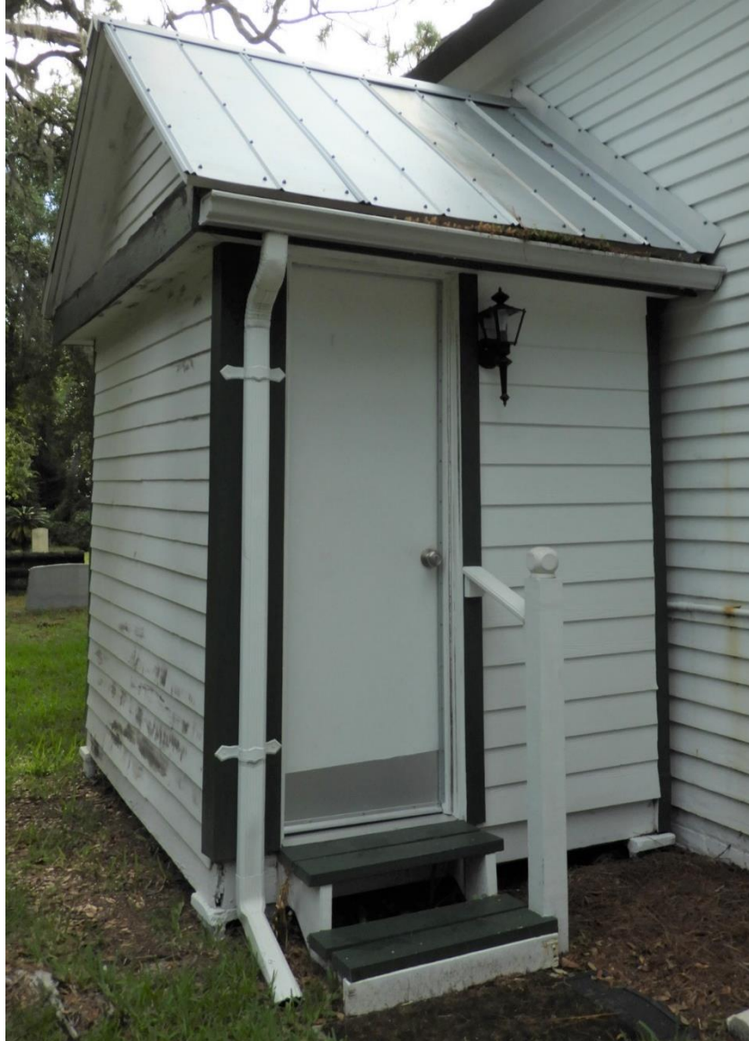
Figure 6 Non-historic alteration/addition with bathroom was added in 1985. The addition is somewhat inconspicuous, as it does not face the roadway.
