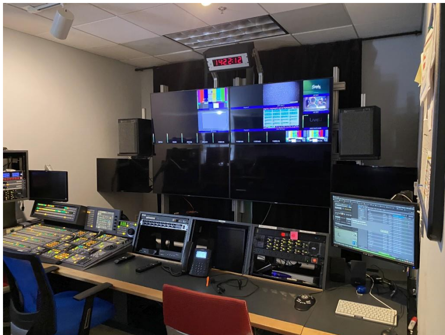
Control Room A
