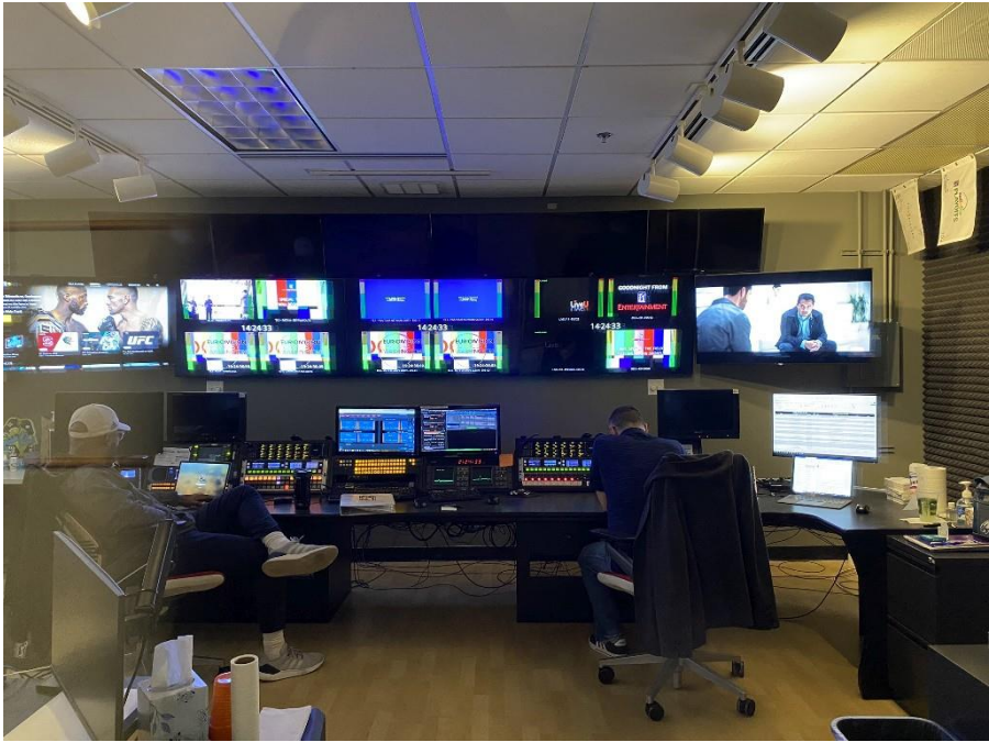
Transmission operations room.
