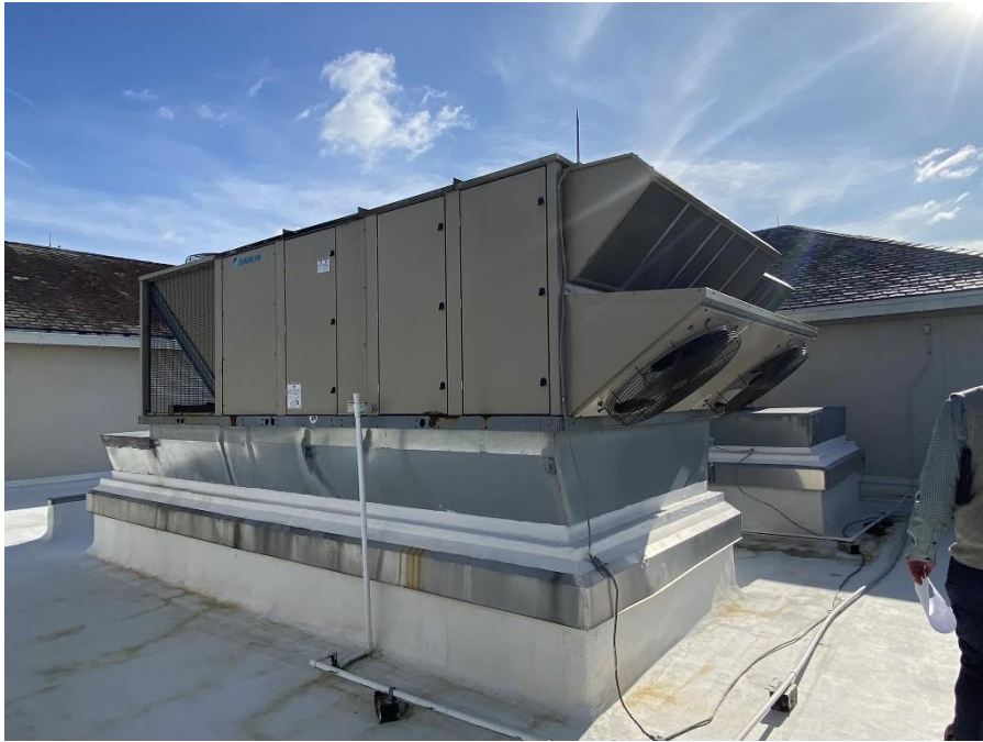
Roof mounted HVAC
